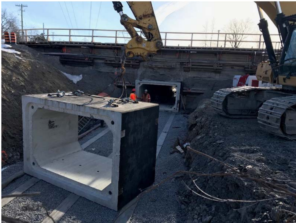
Placing precast box culvert sections on steel grillage for VIA culvert construction.
